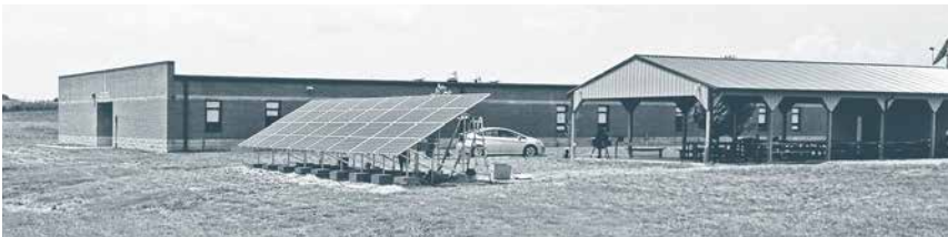
Figure 1.3. This solar array was installed at the Owensville Middle School in Owensville, Missouri, by the author and his business partner, Tom Bruns, and numerous hard-working students. The array is small for a school of this size, which uses almost 1,000 kilowatt-hours per day; the array only provides about 12 days' worth of electricity to the school. The array is also used for science and math education. Credit: Dan Chiras.
