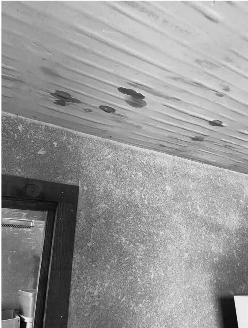
Fig. 1.6: Water is starting to find a way through this green roof after 10 years.
