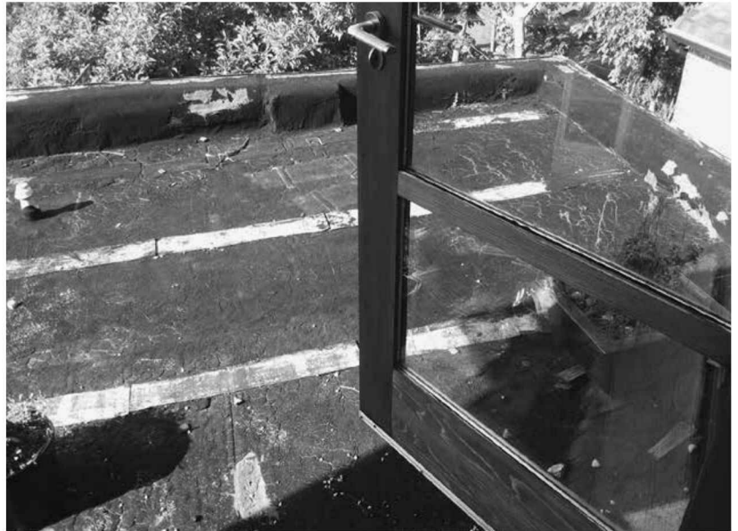
Fig. 1.1: A roof structure gets battered from many exterior forces while protecting precious interiors. PHOTO CREDIT: RESTORATION GARDENS, INC.
