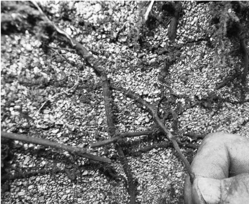
Fig. 2.2: Roots growing within the granules of a typical modified bitumen roof.
