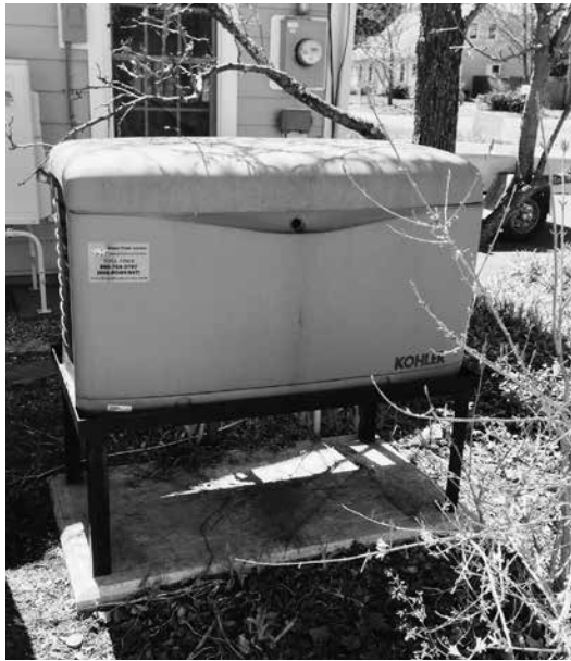
Fig. 1.4: For homes run on critical electric systems, a stand-by generator may be relevant, particularly in rural locations or areas where grid power is less reliable.
