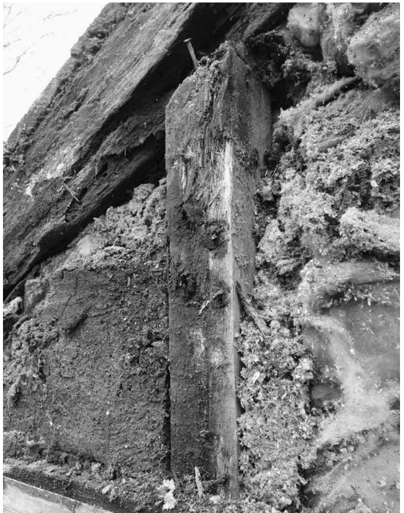
Fig. 1.3: Building physics is at play whether we understand it or not — the penalty for ignoring the physics can be severe! CREDIT: TOP AND BOTTOM RIGHT: NEW FRAMEWORKS NATURAL DESIGN/BUILD.
