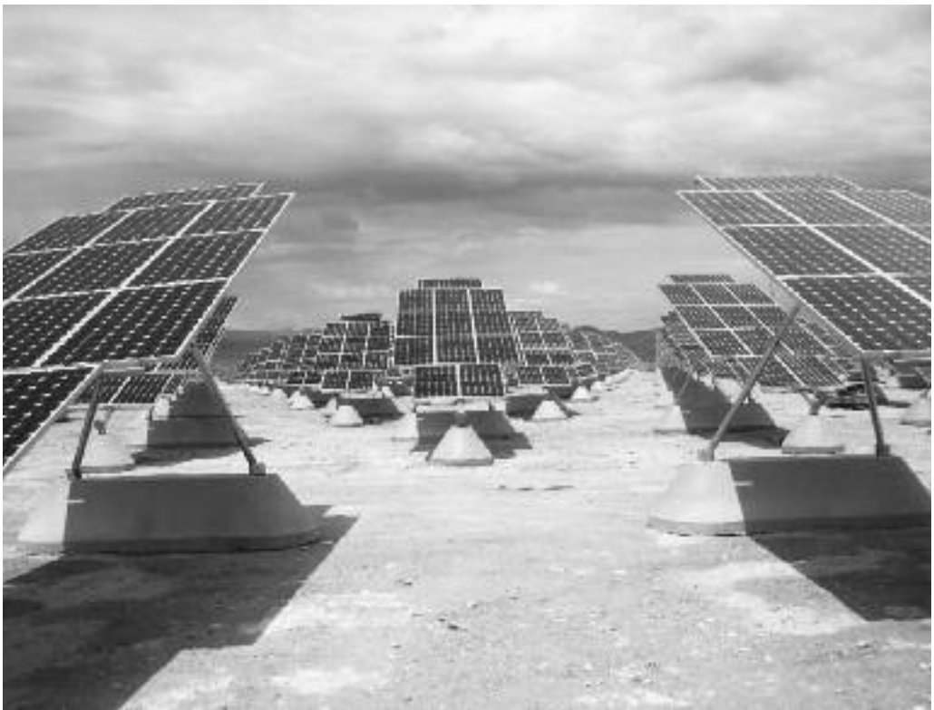
Fig. 1.6: Solar Array. In a renewable energy economy, large-scale solar electric installations, like this one, will supplement electricity produced by other renewable resources, including wind, hydropower and biomass, as well as conventional fuel sources.
